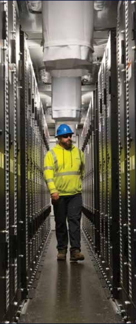
NYPA North Country Energy Storage Facility O'Connell Electric Company
