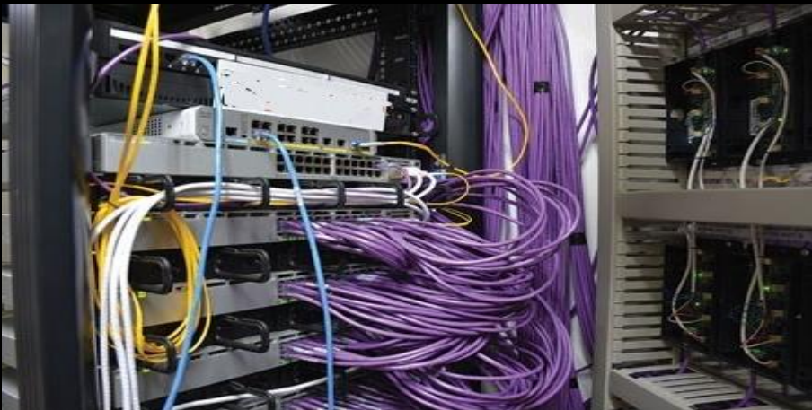
West Baden Springs Hotel PoE Cabling: 500 Lights, 220 Control Nodes
