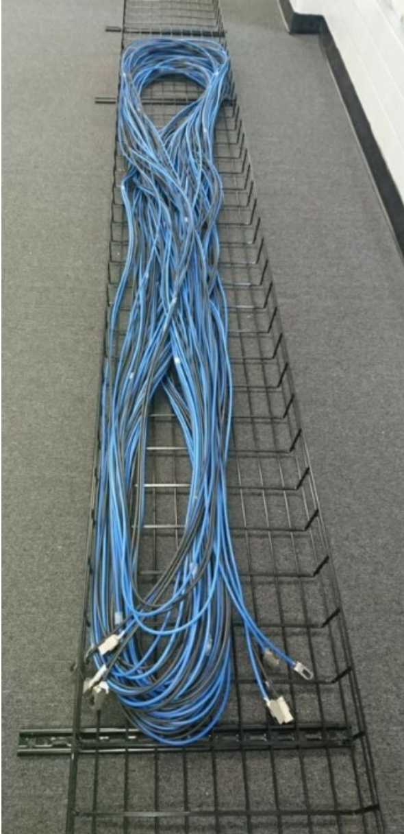
Figure 7. Cable loose in cable tray (not bundled), prior to connecting the field-terminated jacks to the patch cords with factory-terminated plugs.
