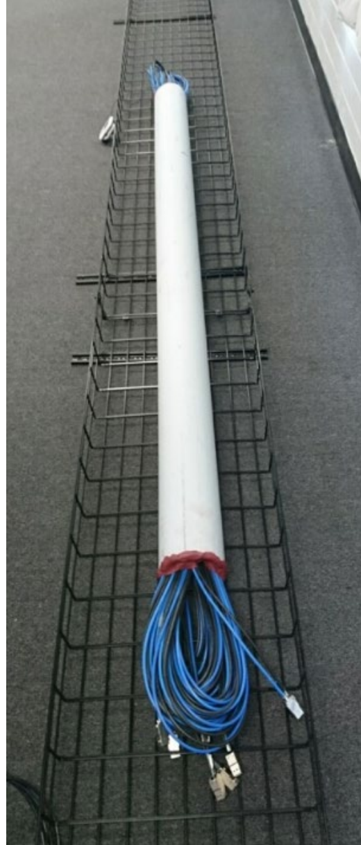
Figure 8. Cable bundled in Schedule 40 PVC conduit, prior to connecting the field-terminated jacks to the patch cords with factory-terminated plugs.
